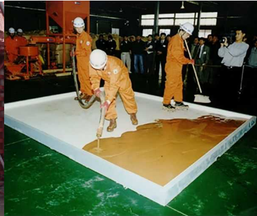
Self-levelling earth (Uni Mkopo), South Korea
